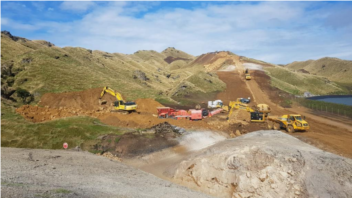
Figure 2: Image of Mobile Aggregate Crusher during construction of the Harapaki wind farm
